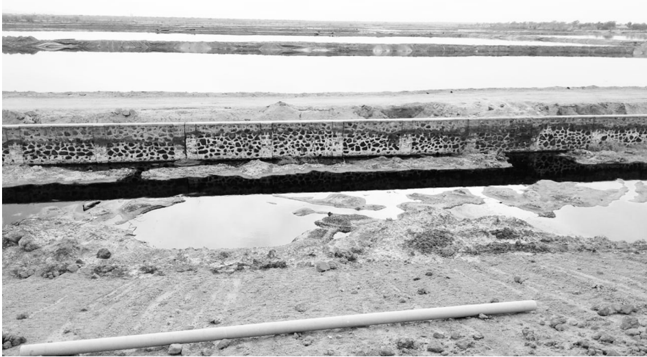
Plate 1- Leakage of partially treated waste water from HRTS walls Source: Field survey. 2019
